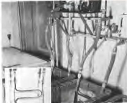
The System Hook-up
