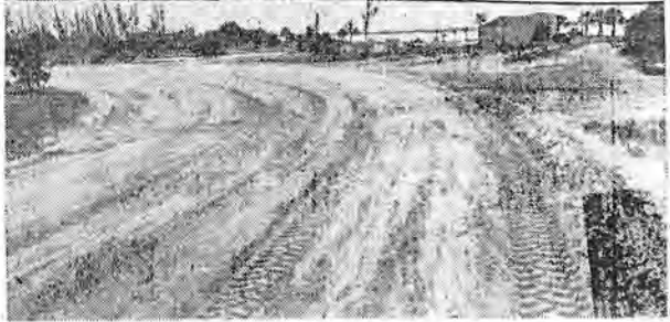
Trotters will get winter training work outs on this dirt track constructed for Wehle by Cleary Brothers of West Palm Beach.
